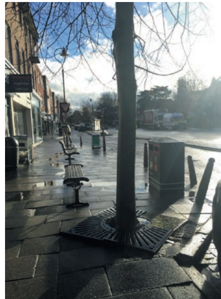
Figure 16a: Radlett District Centre | Cluttered and tired / uneven paving
